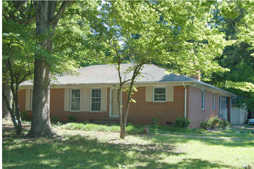
Figure PN-1 - Photograph of the one-story house with instrumented interior drywall crack
