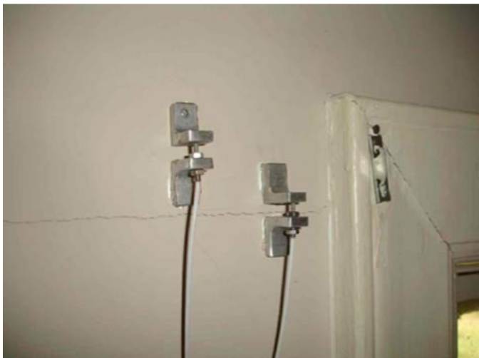
Figure PN-5 - Photograph of interior drywall crack and sensors.
